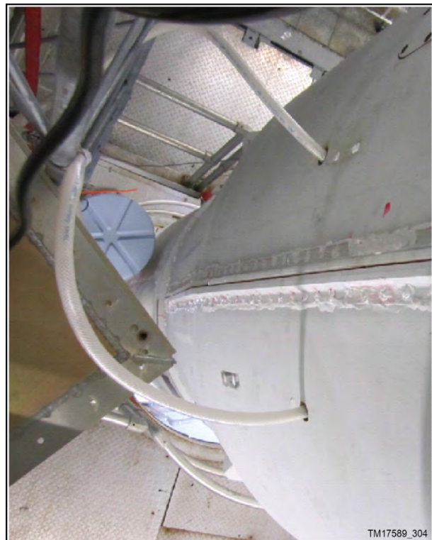
Figure 8.3-1. \text{GN}_2 Purge Interface To Minotaur Fairing (Flyaway at Liftoff)
